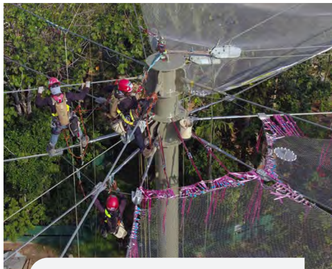
Expert rope accessors take on the tedious and dangerous job of tensioning the pieces of mesh together over the cables.
